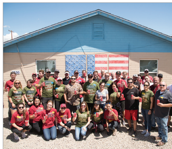
THE D-BACKS TEAMED UP WITH HENSLEY BEVERAGE, BUDWEISER AND REBUILDING TOGETHER TO HELP RENOVATE APARTMENTS FOR HOMELESS VETERANS AT VICTORY PLACE IN DOWNTOWN PHOENIX.
